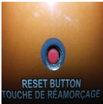
FIGURE 04. HIGH LIMIT RESET THERMOSTAT (LOCATED UNDERNEATH).
